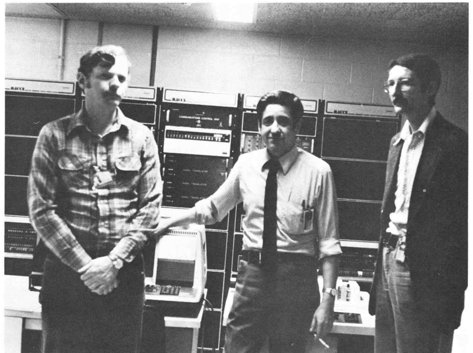
Hernan Otano (center) is Chief of Audio-Visual Systems at the National Air and Space Museum. With him are Dick Wakefield (left) and John Hartman. They are shown in the control center which contains a PDP 11/40. The 11/40 monitors each audio-visual installation plus much of the track lighting. This continuous monitoring takes 34,000 operations, performed at five a second. The 11/40 also starts the exhibits in the morning and shuts them down at night. Otano says in the six years of operation, they have only had 1/2 hour of down time.
