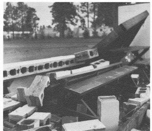
PATIO WALL at the IO building toppled over at 5:30 Friday evening during the first part of the windstorm. Picnic table was destroyed.
